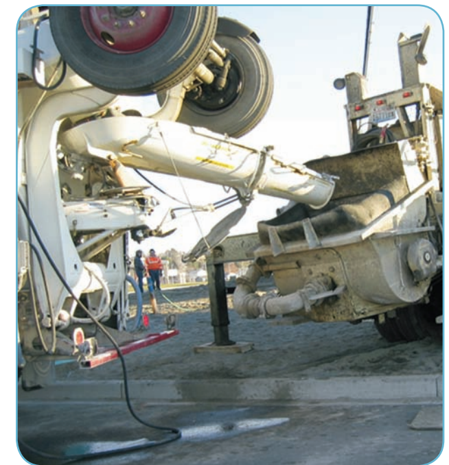
Potential for concrete to spill into gutter.
