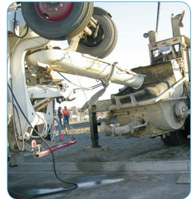
Potential for concrete to spill into gutter.
